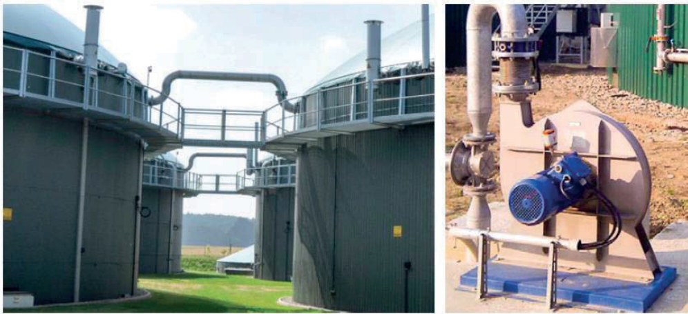
Figure 6. Working platforms between tanks with pipelines and pressure adjustment devices (left); gas compressor (right).
