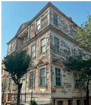
Figure 6. Deterioration of wood.
