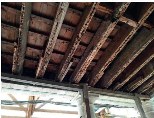
Figure 1. Moisture and insect-damaged wooden beam.
