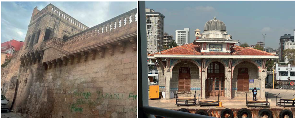
Figure 12,13. Damage to historical structures from environment and human intervention.
