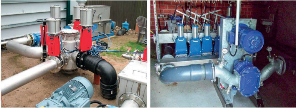
Figure 5. Pipelines and fittings in the pumping station, shut-off valve.
