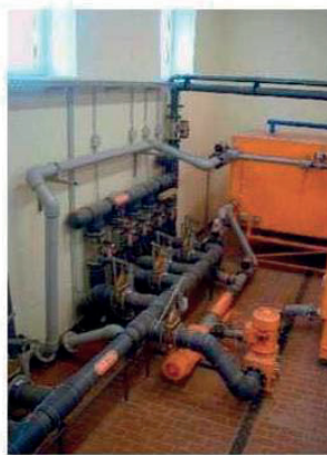
Figure 2. Pumps in the biogas plant.
