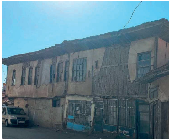
Figure 7. Deterioration of plaster and wood.
