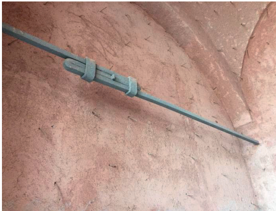
Figure 10. Repaired iron deterioration.
